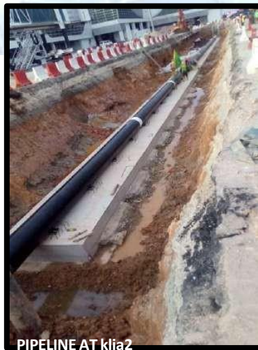
PIPELINE AT klia2
